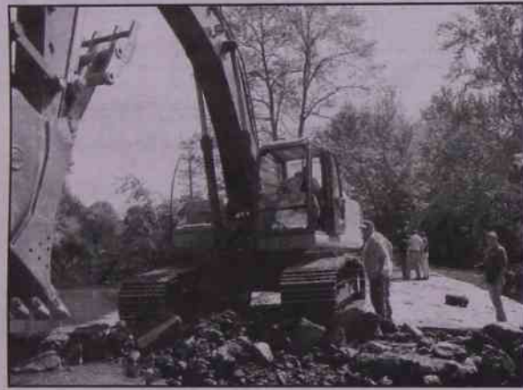
Doug Hall removes a portion of the Nashville Dam's cap while Chris Freiburger and David Kenyon of the Michigan DNR look on.
