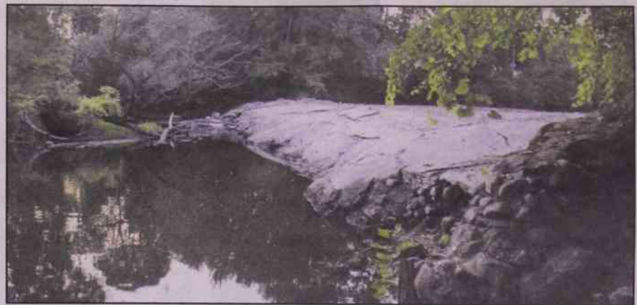
Work has begun on the removal of the Nashville Dam. Demolition will continue during the upcoming week.
