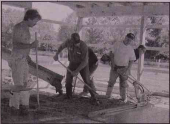
Volunteers pour cement into the floor of the pole barn. The barn will be a secure, weather-proof building to store equipment used to maintain the cemetery.
