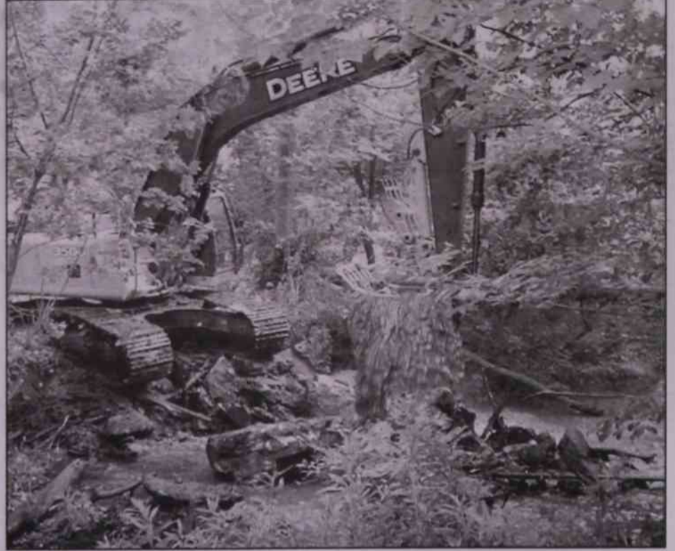
DNR construction crew works to remove remnants of the Maple Hill Dam on Butternut Creek in the Thornapple River Watershed.
