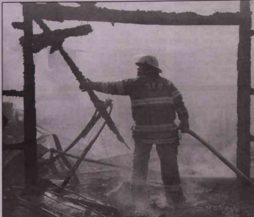
Working to make sure the rest of the wall is stable, a Sunfield firefighter works to remove some of the burned rubble.
