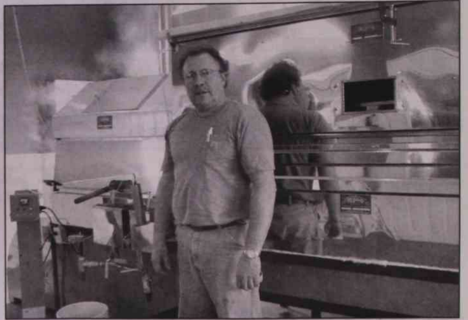
Brian Benedict stands next to his new boiler system that allows him to reach a higher level of efficiency and draw twice the amount of syrup for the same amount of fuel as his previous system.
