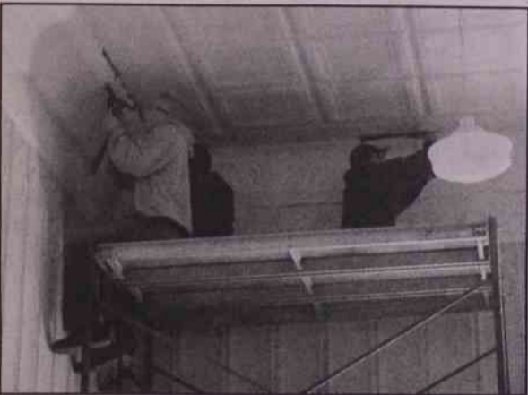
Levi Westendorp, Sean Curtis and Justin Kennedy work to carefully peel tin panels from the ceiling of the old Masonic lodge in Nashville. The building is now home to The Revue theater group.
