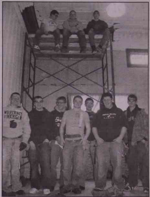
Students of Jeff Seavolt's building trades class at Maple Valley High School take a moment to pause for a picture on the stage they have been working on. Shown here are (from left) Dylan Myers, Brogan Bodemuller, Brandon Hoffman, Jesse Miller, Tyler Murray, Matt Turner, Mark Wehr, (on scaffolding) Sean Curtis, Levi Westendorp and Justin Kennedy.
