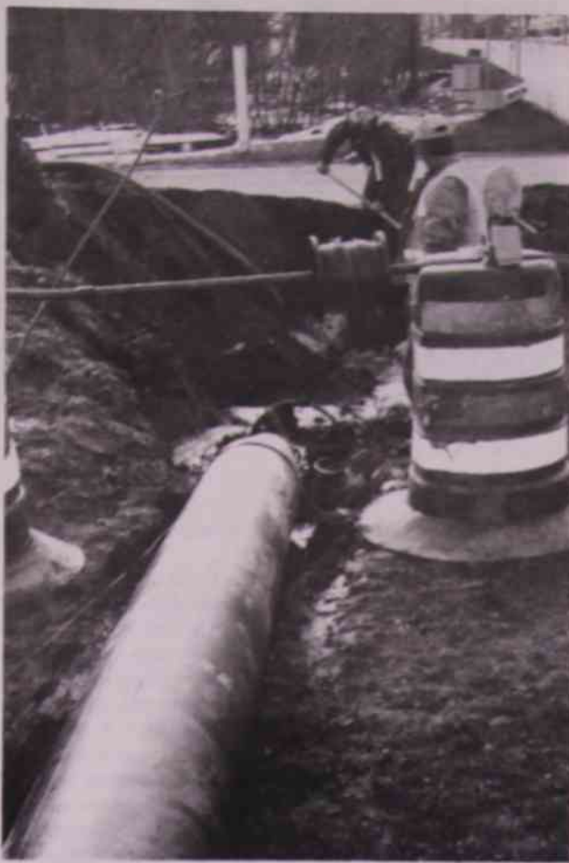
In July work was still in progress on the Reed Street reconstruction project.
