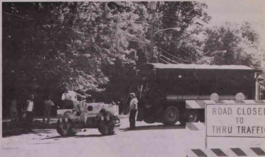
In July work was still in progress on the Reed Street reconstruction project.
