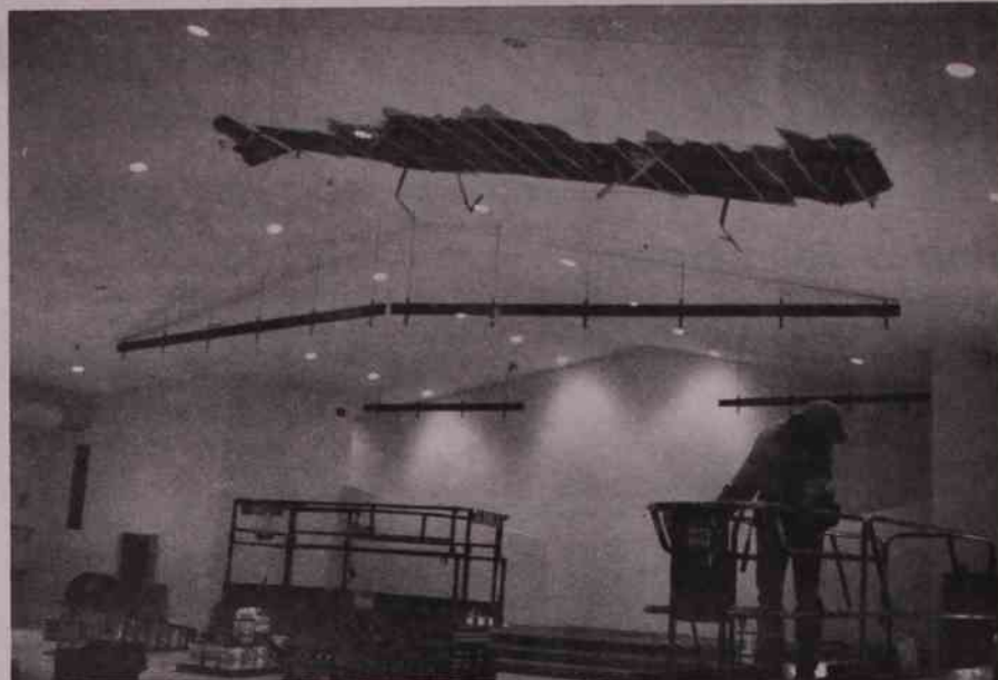
Work continues inside the auditorium at the new Grace Community Church despite damage caused to the ceiling and rafters by a smoldering fire.
