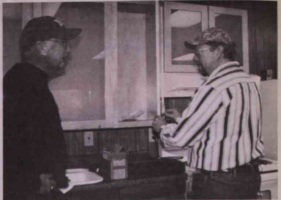
Maple Valley Alternative Education Principal Tate Mix looks on as Kim Hansen from the Maple Valley Schools maintenance department installs hardware on the kitchen cabinets in the new life skills center at Kellogg School in Nashville. Not pictured is Steve Augustine, from the Maple Valley Schools maintenance department.
