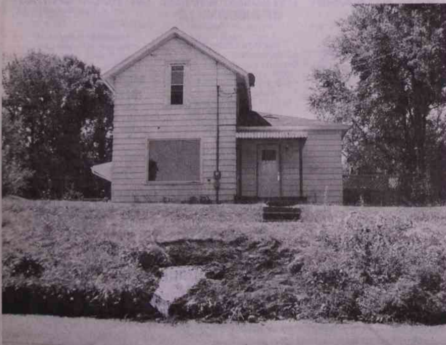
The embankment was sheared and the Casgrove Street house (in background) was damaged when a pickup truck left the roadway and crashed Aug. 7.
