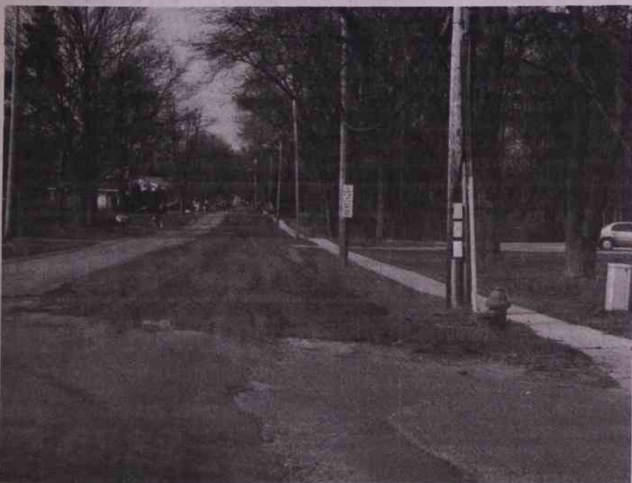
Construction has started on Reed Street, and will not be completed until sometime around September. With the street being repaired, and the water mains all over town being replaced Nashville will face traffic woes.
