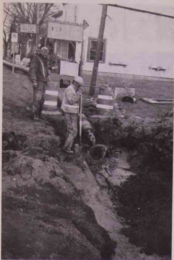
Work has gotten underway on the Nashville water project. Here, workers from West Michigan Cable do some directional boring.
