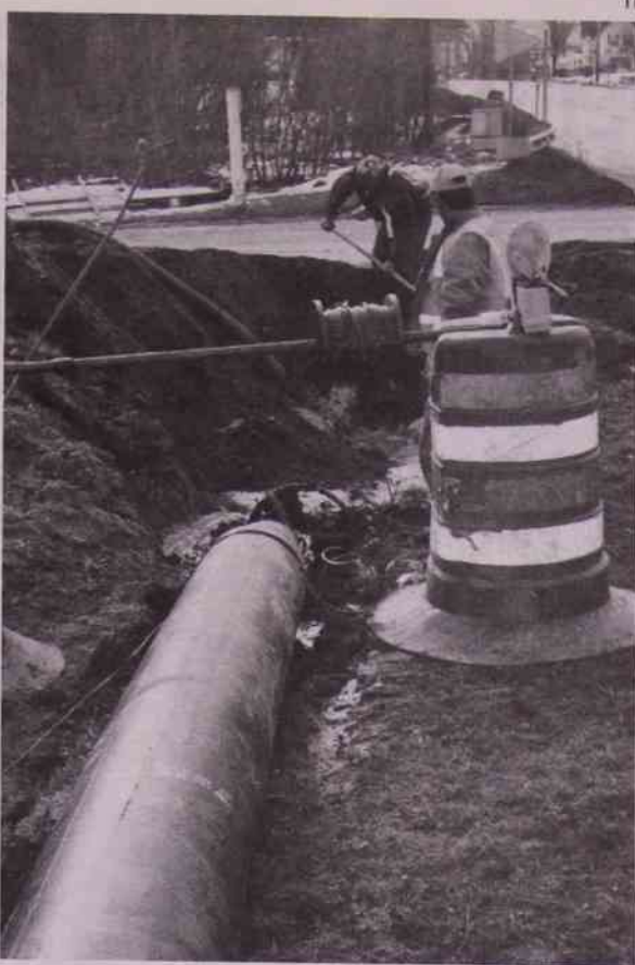
The Nashville water project work was being done last week, workers were boring in holes to install 12 inch water main that started at Frances Street and went to Railroad Street.
